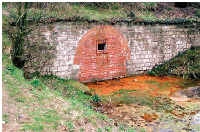
The west portal of Norwood tunnel in 1978. Through the bars it is possible to see that the tunnel roof has collapsed within a few metres. Photo Nick Catford
